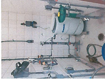
AME Well chlorination room
