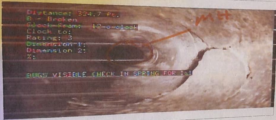
Broken Sewer Line
